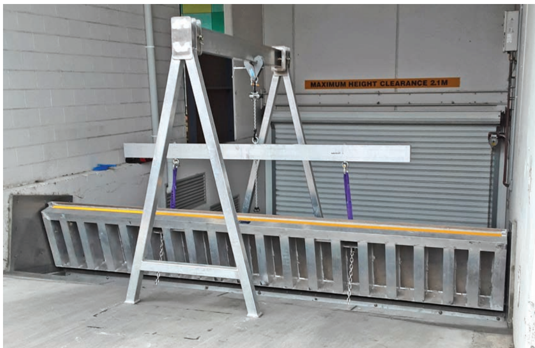
Figure 17: Example of a permanent buoyant tilting flood barrier during a routine maintenance check
