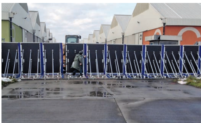
Figure 7: Example of a temporary demountable flood barrier protecting a factory complex
