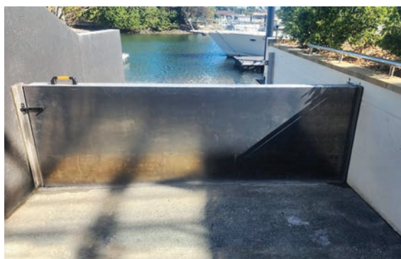
Figure 5: Examples of manually operated flood barriers
