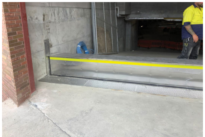
AWMA Flood Barrier deployed in the Ballarat GovHub basement carpark.
